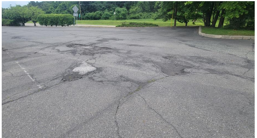
Photo 3 – Deteriorated Asphalt Parking Lot
